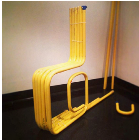
pic 3. The pipe are not level
